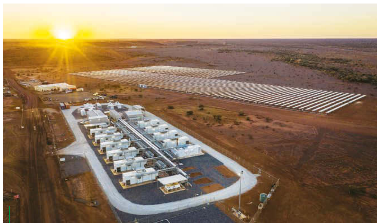
EDL's hybrid renewable microgrid at the Agnew gold mine in Australia successfully demonstrates the potential for renewable energy with storage in the mining sector.
