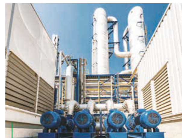
AVR's carbon capture plant in Duiven, Netherlands, makes greenhouse horticulture more sustainable while putting CO 2 emissions to productive use.
