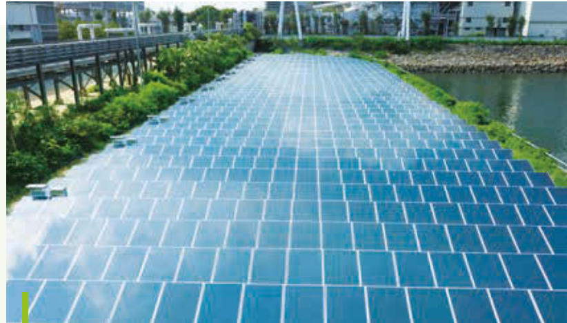
Solar power facilities at HK Electric's Lamma Power Station.
