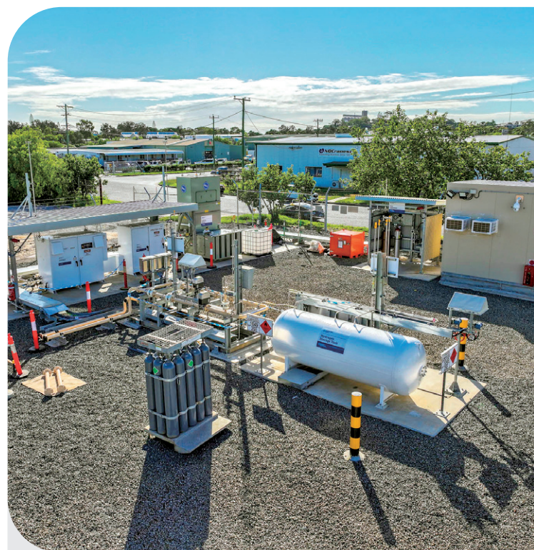
➤ Hydrogen Park Gladstone, AGN's renewable hydrogen production facility in Queensland, Australia, is helping to decarbonise the company's gas supply with an electrolyser that uses water and certified renewable electricity.
