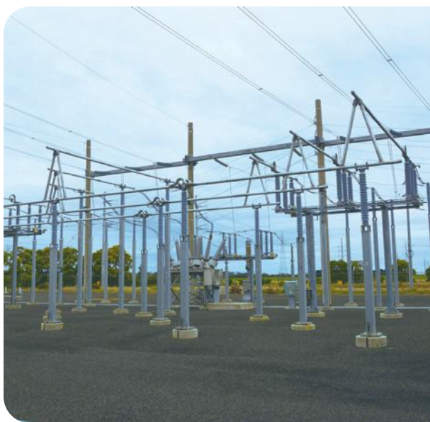
▶ AEO's network infrastructure connects more than 800 MW of wind energy to the grid.
