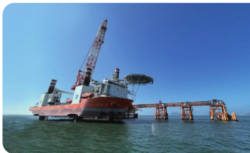
▶ The construction of an offshore liquefied natural gas terminal in Hong Kong reaches critical milestones. It will enable the import of natural gas through marine routes.
