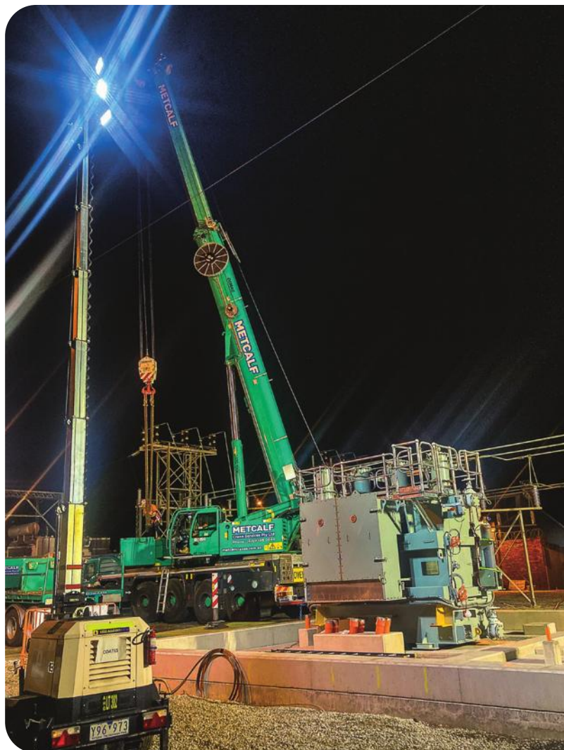
UE completes a major upgrade to the Sandringham Zone Substation as part of a multi-million network enhancement project.
