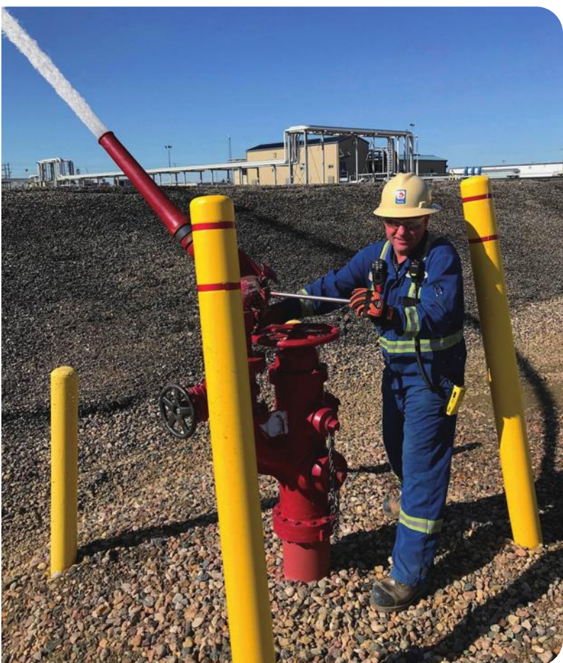
▶ To ensure asset and employee safety, an expert working for HMLP demonstrates fire prevention procedures at Lloyd Terminal.
