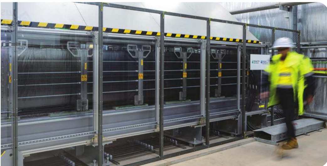
AGN's zero-emissions 1.25-MW electrolysis plant in South Australia creates green hydrogen and enables completely zero-carbon heating.
