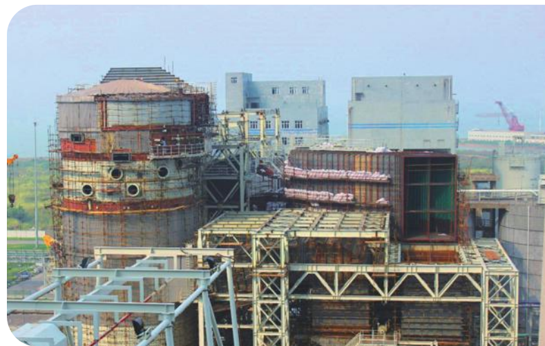
The Jinwan Power Plant's maintenance and repair programme minimises emissions while maintaining performance.
